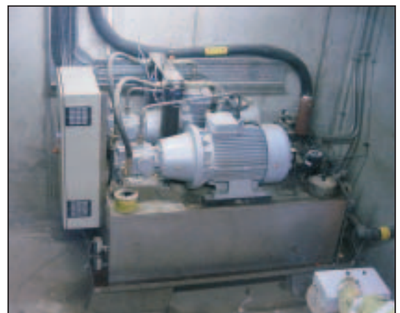
The Hydraulic Power Pack
